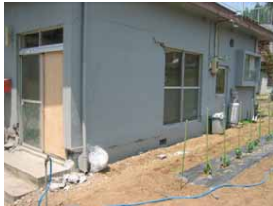
Photo 16 Damage to concrete-block masonry structure
