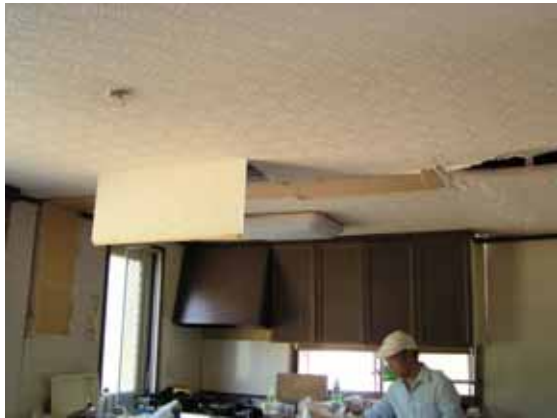
Photo 15 Fallen storage facilities in kitchen
