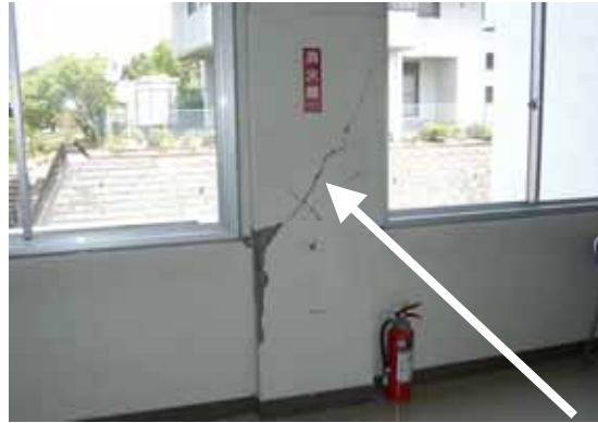
Photo 10 Shear cracking to the Second floor columns of the old building
