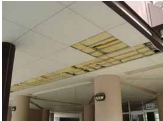
Photo 8 Fallen ceiling panels at front entrance
