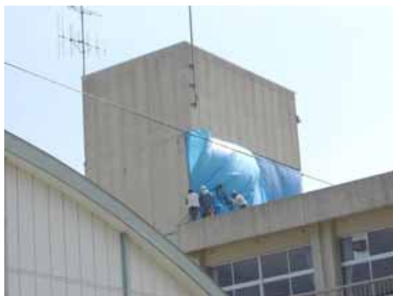
Photo 17 Damage to steel frame tower on roof
