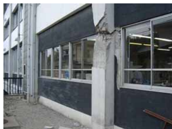
Photo 5 Shear cracking on the columns beside the entrance
