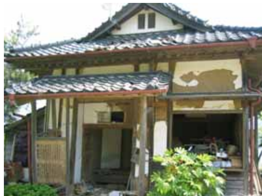
Photo 12 Damage to outer wall of one-story wooden residence
