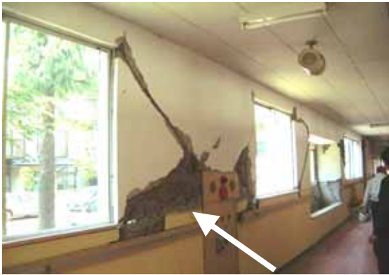
Photo 7 Damage to the wall between openings in the first floor corridor of the old building
