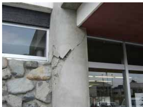
Photo 6 Damage to the columns at the rear of the main building
