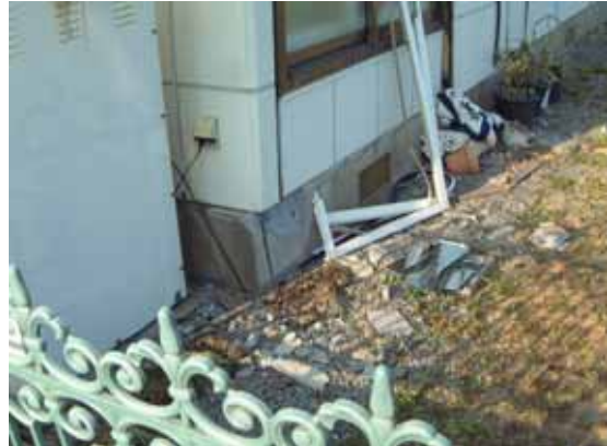
Photo 14 Damage to lightweight steel frame prefabricated residence
