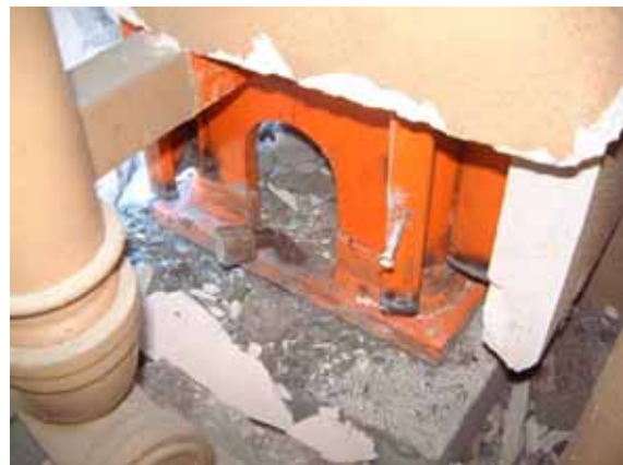
Photo 18 Rupture of foundation anchors on tower
