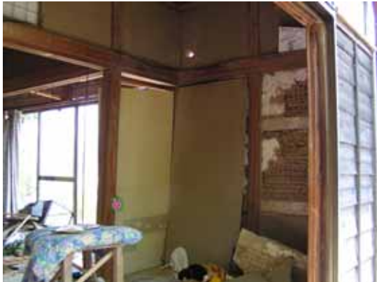
Photo 13 Damage to inner wall of one-story wooden residence
