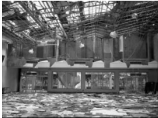
Photo.2 Damaged Roofing Materials of Public Hall (Miyako Island)
