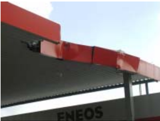
Photo.19 Damaged Roof of Gas Station by Flying Debris (Hachijo Island)
