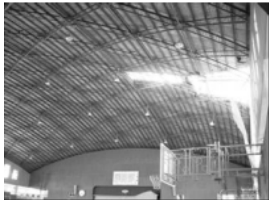
Photo.3 Separation of Roofing Materials of Gymnasium (Miyako Island)
