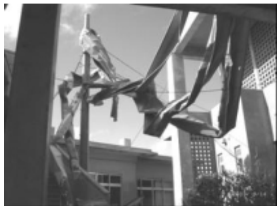
Photo.4 Exfoliation of Roofing Materials of Gymnasium (Miyako Island)
