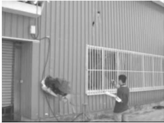
Photo.5 Damaged Wall by Flying Debris (Miyako Island)
