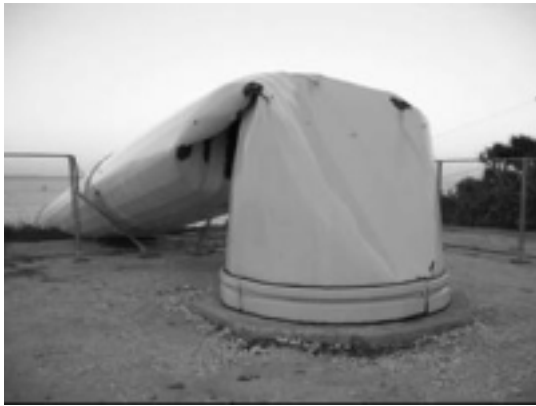
Photo.14 Broken Tower of Wind Turbine Generator System (Miyako Island)
