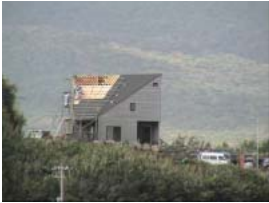
Photo.9 Exfoliation of Roofing Materials on Timber House (Hachijo Island)
