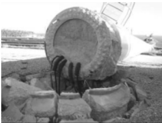
Photo.15 Collapsed Wind Turbine Generator System with Its Footing Pulled Out (Miyako Island)
