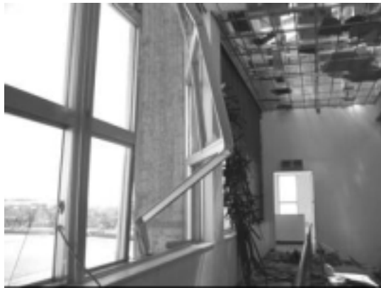
Photo.6 Broken Metal-framed Window and Ceiling Finish Materials of Gymnasium (Miyako Island)
