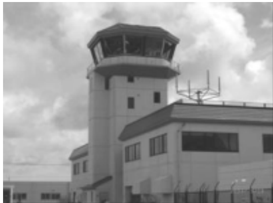
Photo.1 Damaged Windows on Airport Control Tower (Miyako Island)
