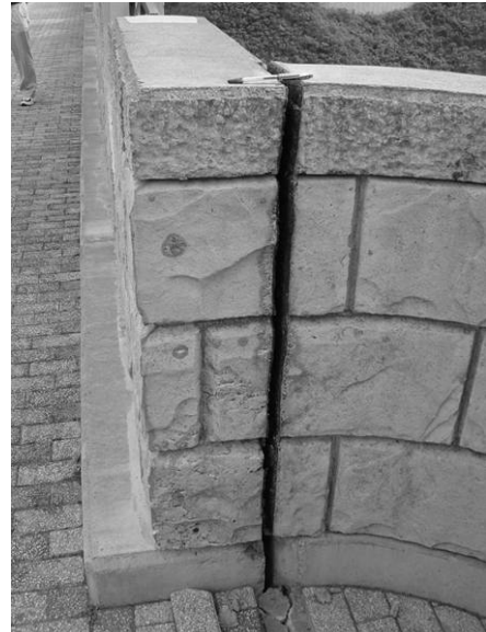
Photograph 2 Opening of Joints on Balustrade (Hinata Dam)
