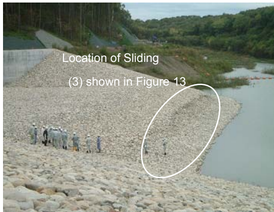
Photograph 9 Sliding of Protective Rock Layer of Makubetsu Dam
