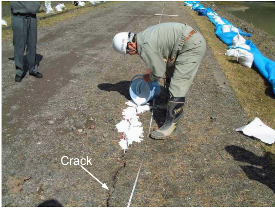
Photograph 5 Crack at Crest of Dam (Takami Dam)
