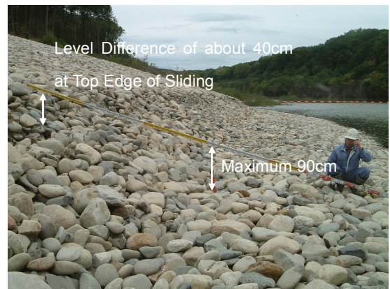
Photograph 10 Sliding of Protective Rock Layer of Makubetsu Dam (Enlargement)
