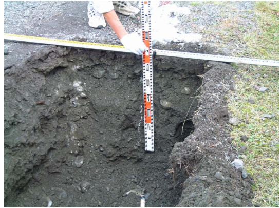
Photograph 6 Survey of Crack Depth by Exploratory Pit (Takami Dam)
