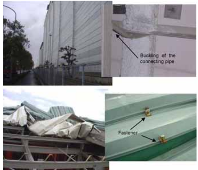
Fig.5 Failure of Large-scale Warehouse at Kobe
