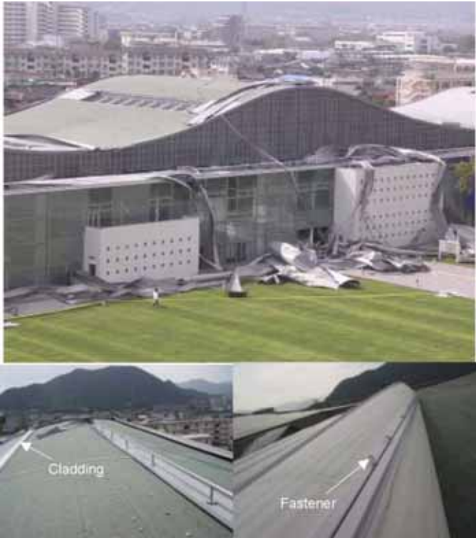
Fig.1 Failure of Roofing Materials of YCAM due to Typhoon 0418
