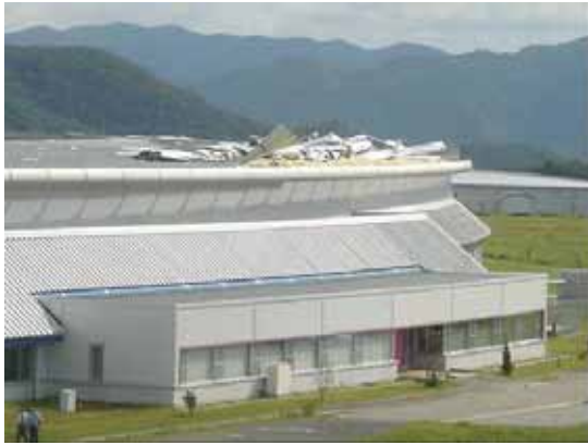
Fig.3 Failure of the roof of SPring 8
