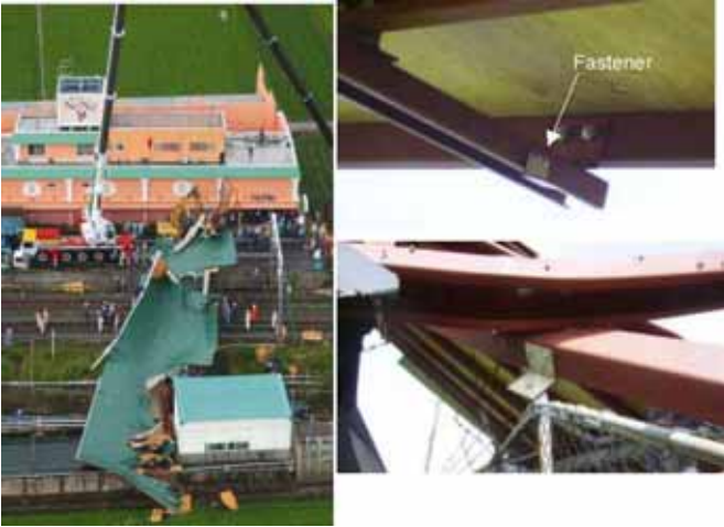
Fig.8 Blown Roofing Material from the Motor Inn
