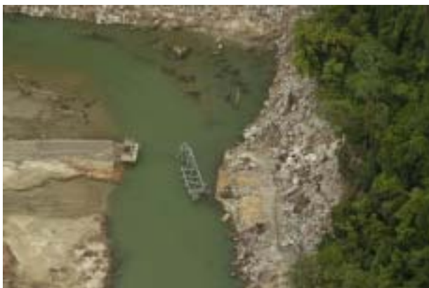
Photo 24 Washout of Truss Bridge (3)
