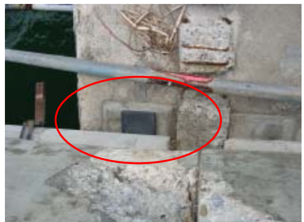
Photo 8 Rubber Sheet Type Bearing and Lateral Displacement at Bearing
