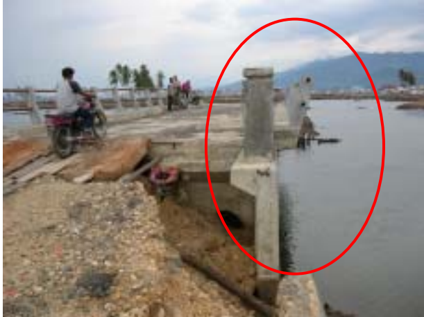
Photo 9 Lateral Displacement of Deck
