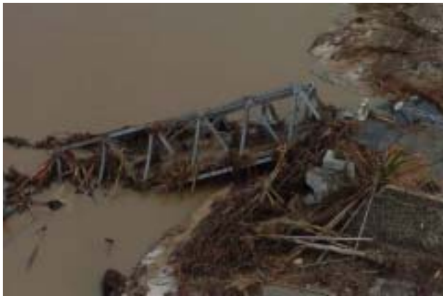
Photo 22 Washout of Truss Bridge (1)
