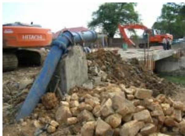
Photo 2 Collapse of Water Pipes Bridge
