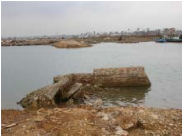
Photo 3 Complete Washout of Bridge (reported as Wooden Superstructure)
