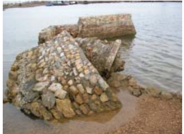
Photo 4 Masonry Substructure and Washout Effect of Surrounding Soils
