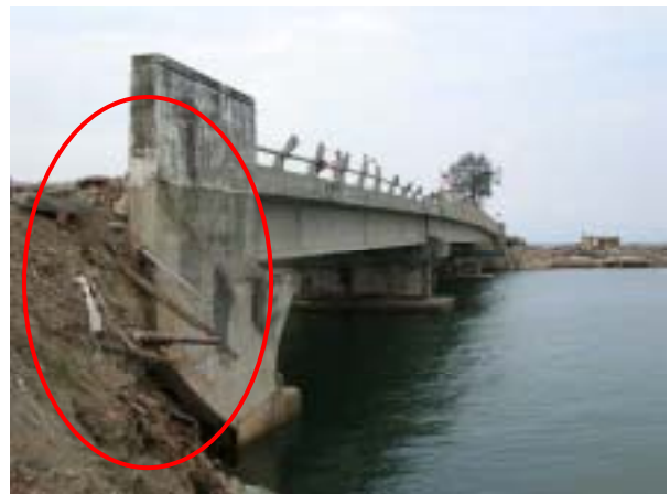
Photo 6 Washout Effect of Backfill Soils
