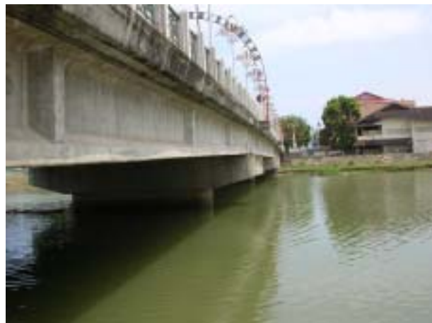
Photo 13 Bridge affected by Shaking
