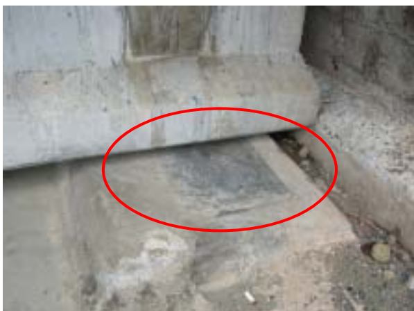
Photo 7 Lateral Displacement of Deck
