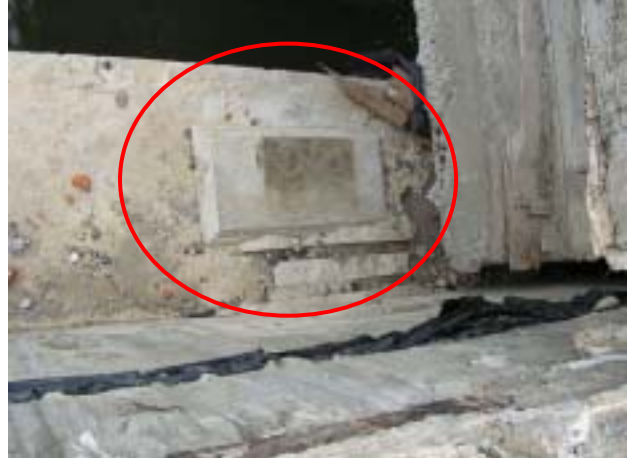
Photo 10 Displacement at Bearing
