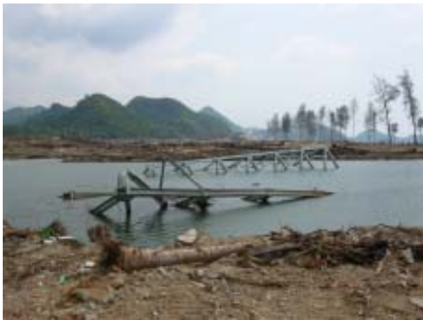
Photo 17 Washing out of Steel Truss
