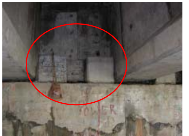
Photo 14 Slight Damage to Shear Keys by Shaking
