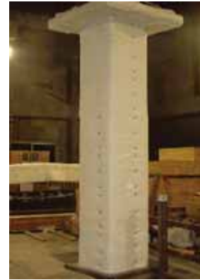
Photo 1. Blanket-type Fire Protection
