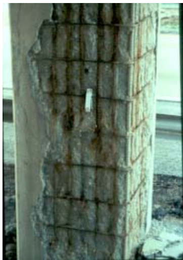
Figure 1. Corrosion Damage to Concrete Bridge Pier
