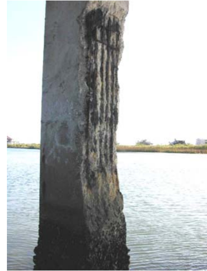
Figure 1: Spalling and rebar cross-sectional loss on a bridge piling due to corrosion.
