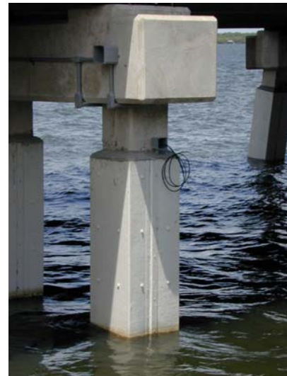
Figure 6: Titanium mesh pile jacket installed at splash zone elevation. The anode is pre-installed in the fiberglass form then placed around the pile and filled with mortar/concrete.
