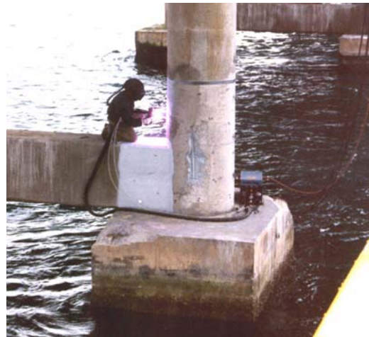
Figure 8: Arc-sprayed zinc applied to the concrete surface to produce the cathodic protection current.
