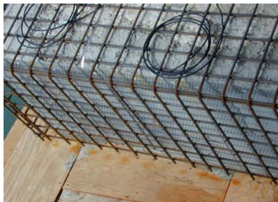
Figure 5: Titanium mesh anode installed over original concrete to be encapsulated in structural concrete.
