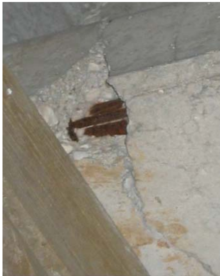
Fig. 9 – Corroded strands at crack location.
