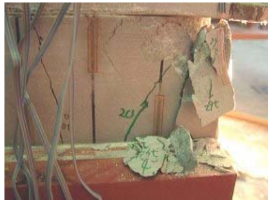
Figure 15. Crushing of supporting mortar in overhang type specimen [North connection, Back side]
