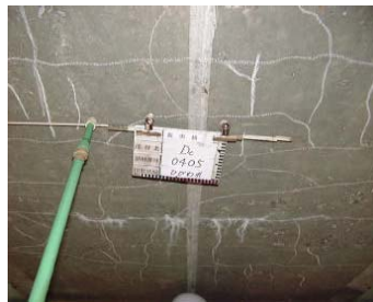
(a)cracks on RC slab
