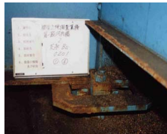
(b)corrosion in bearing
