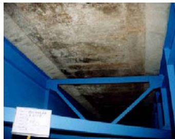
(a)cracks on RC slab
