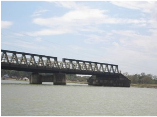
Figure 4a. Supporting piers of Arugam Bridge in Sri Lanka shifted due to foundation Scour in the Dec. 2004 Indian Ocean Tsunami.
