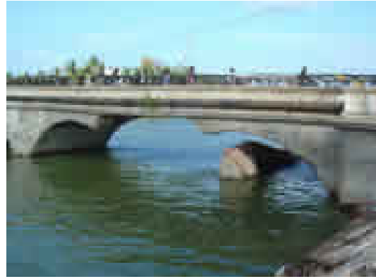
Figure 4b. Collapse of pedestal of the Karaikal Bridge in India due to scour in the Dec. 2004 Indian Ocean Tsunami.
