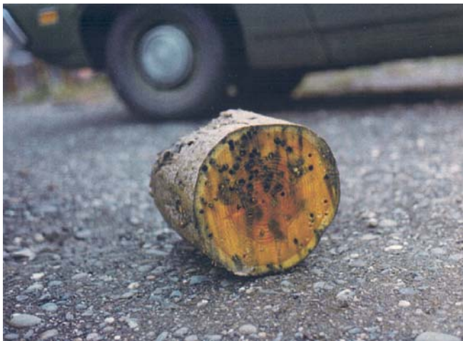
Photo 3 – Marine Borer damage to timber pile at Pier 2.
