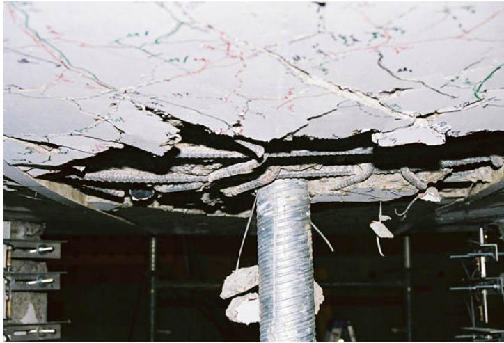
Figure 4 - Straightening of 90° J-hook at the end of test of Unit-1
