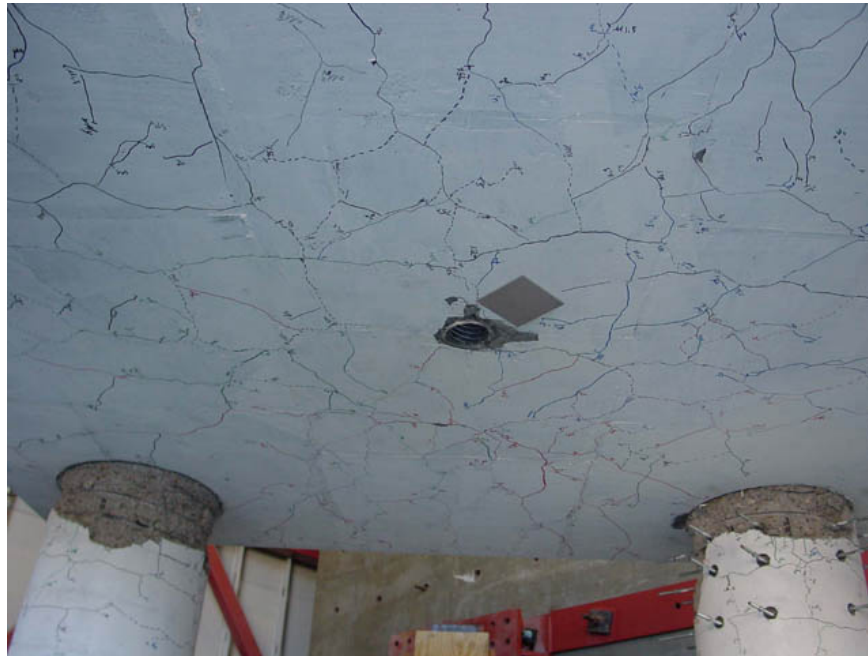
Figure 6 - Pilecap soffit at the end of test of Unit 2
