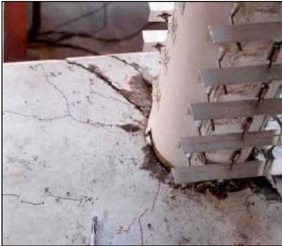
Figure 3 Pile Cap Damage in the Anchorage Region
