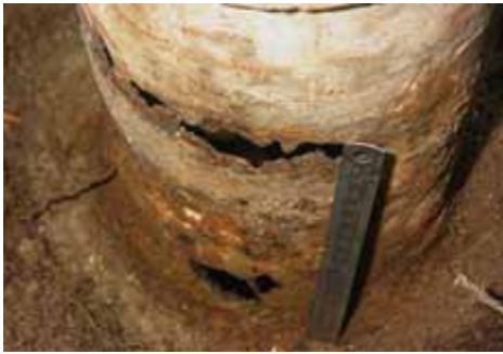
Photo 2 Light pole corrosion
