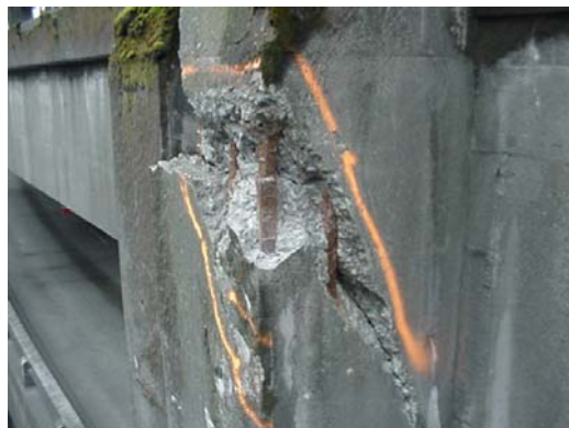
Figure 2, Damage to Bent 100, East Column, Upper Deck Joint
