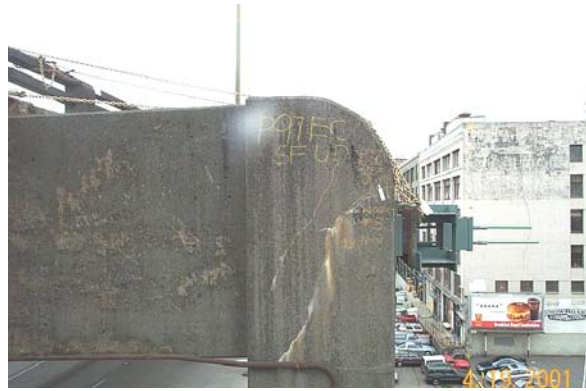
Figure 3, Damage to Bent 97, East Column, Upper Deck Joint
