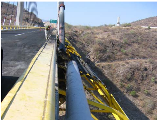
Mezcala Bridge – Fire and Cable Failure
