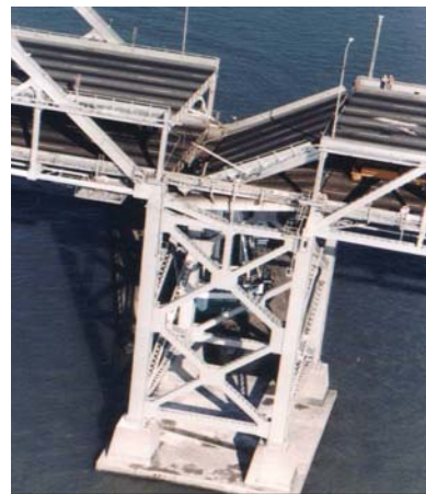
FIGURE 1: PIER E9 DAMAGE FROM THE LOMA PRIETA EARTHQUAKE
