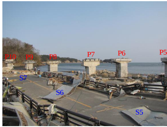
Fig. 13 General damage to piers
