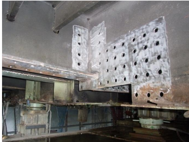
PHOTO 3 GIRDER G7 IMMEDIATELY AFTER REMOVAL OF THE PARTS WITH CRACKS
