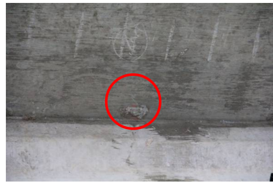
FIG. 17: AFTER HAMMER SOUNDING
