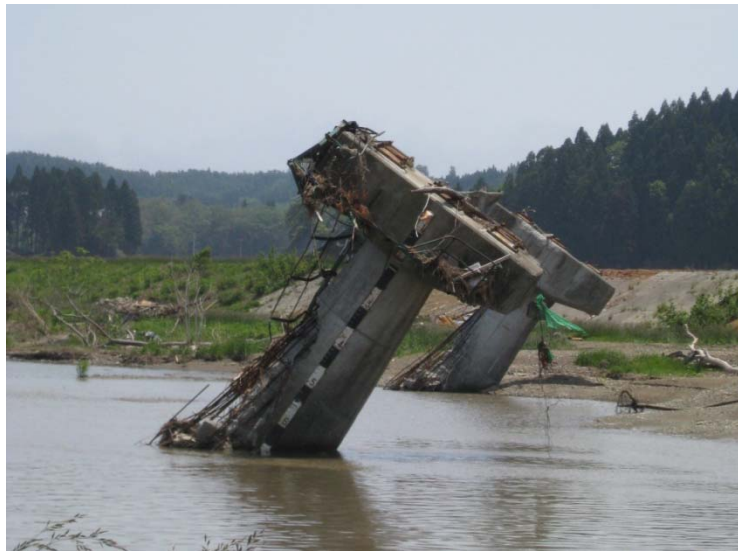
FIGURE 2. DAMAGED PIERS OF THE JR RAIL VIADUCT CROSSING THE TSUYA RIVER, TOHOKU EARTHQUAKE, 2011 (PHOTO: S. DASHTI)
