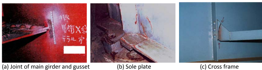
Figure 4. Cracks at different positions in steel superstructures
