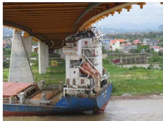
Figure 2 Ship Collision of Main Girder
