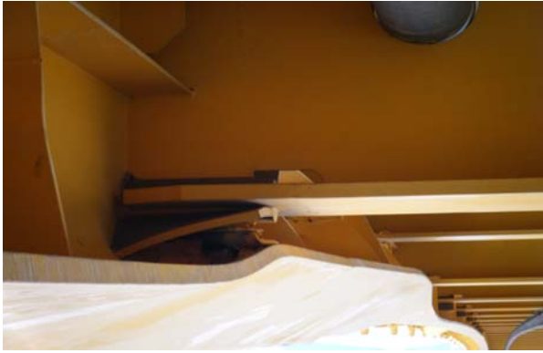
Figure 4 Damaged Edge Girder (Inner side)
