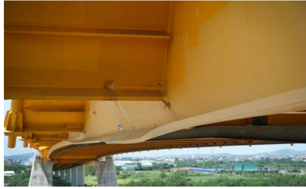
Figure 5 Damaged Edge Girder (Outer side)
