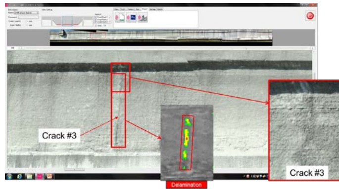
Fig.11: Typical cracks with delamination on the reinforced concrete bridge railing
