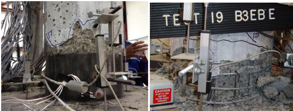
Fig.7. Damage comparison between the new bridge system and conventional bridge after test 19. (Right figure from test 19 of conventional bridge (Johnson et al., 2006)
