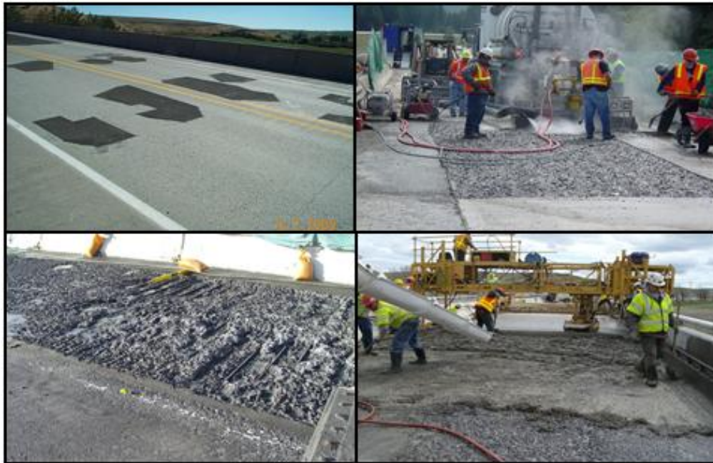
Figure 5: Bridge Deck Deterioration
