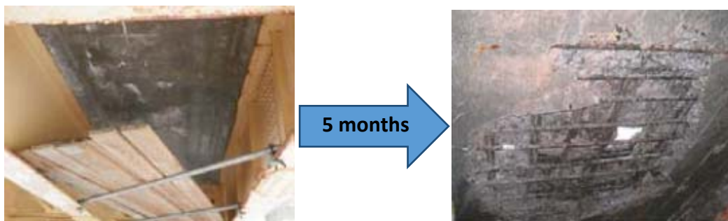
FIGURE 1 An example of the collapse of an RC deck having only minor cracks
