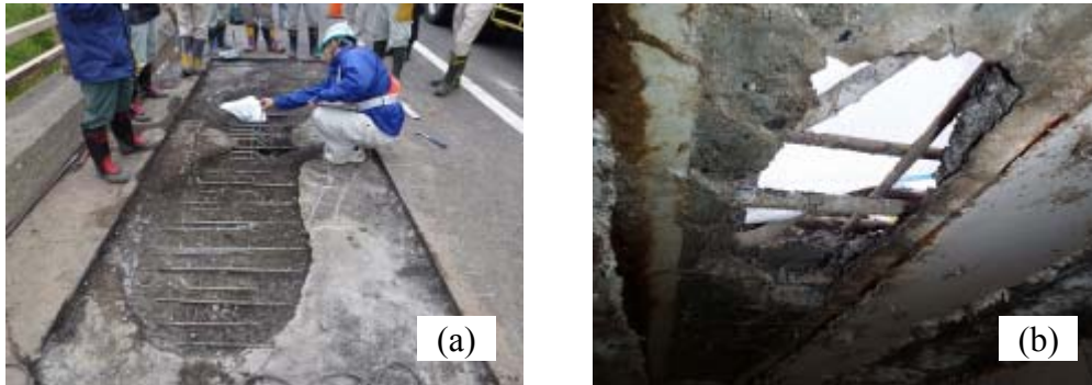
Figure 1 PARTIAL COLLAPSE OF RC SLAB IN HOKKAIDO: (a) damage condition on top surface; (b) view from bottom surface
