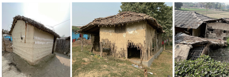
Photo 2: Affected temporary houses by a flood event of 2024 in the Bagmati River basin, Nepal
