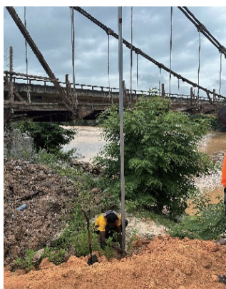
Photo 3 Installation of a fixed-point camera for continuous water-level and discharge monitoring
