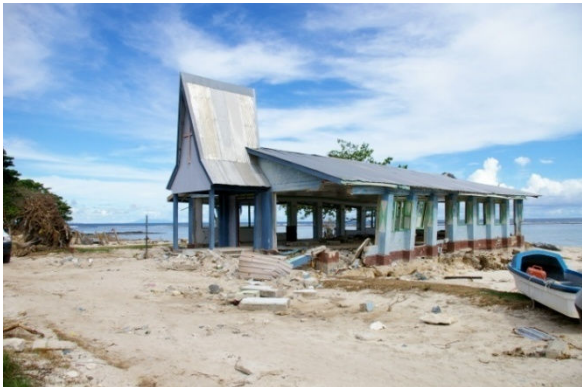
A church in Ghizo Island damaged by Solomon Tsunami in 2007
