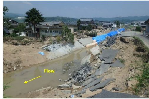
Photo 4-2 Levee breach along the Suemasa River (Mabi Town, Kurashiki City)
