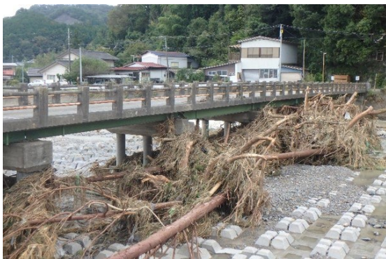
Photo 4-3 Driftwood accumulated at Tokiwa Bridge
