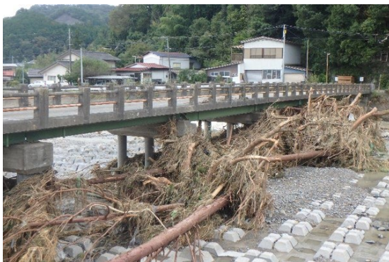
Photo 3-3 Driftwood accumulated at Tokiwa Bridge
