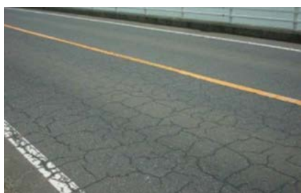
Figure 3: Pavement surface cracks due to asphalt deterioration
