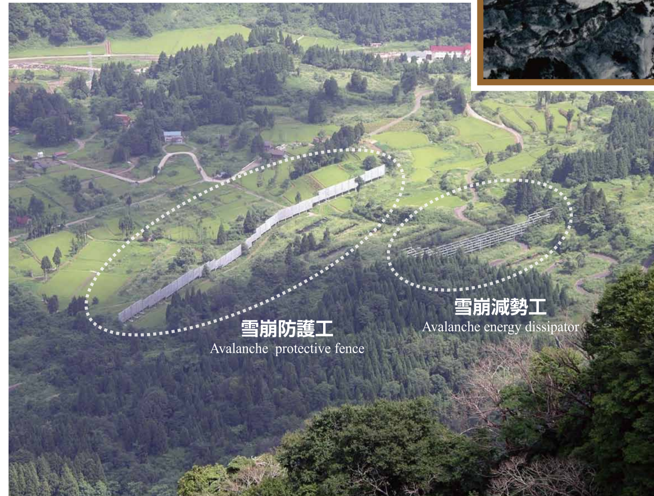
▲柵口の集落を守る雪崩減勢工、雪崩防護工 The energy dissipating structure and the avalanche-protection structure in the Maseguchi district
